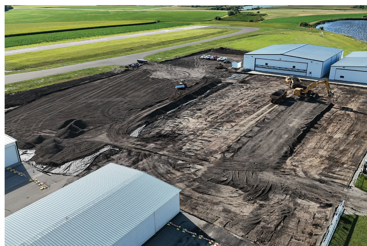
Apron expansion increases parking, reduces congestion, and improves ground handling (under construction).
