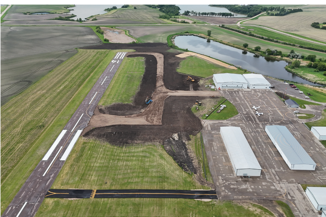
A temporary taxiway maintained FBO access and kept operations running during taxiway upgrades.
